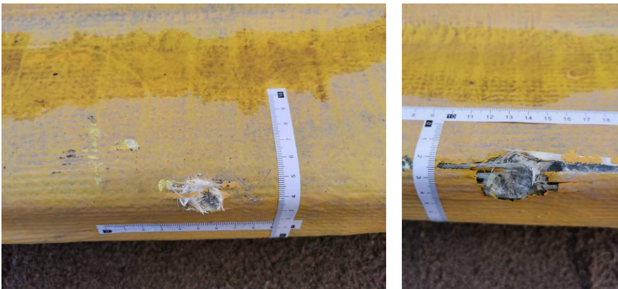
Figure 4: Damage of the Protective Cover
