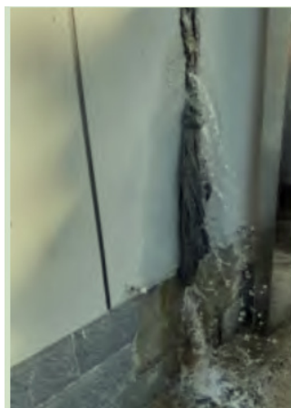
Figure 1: Expansion joint leakage
